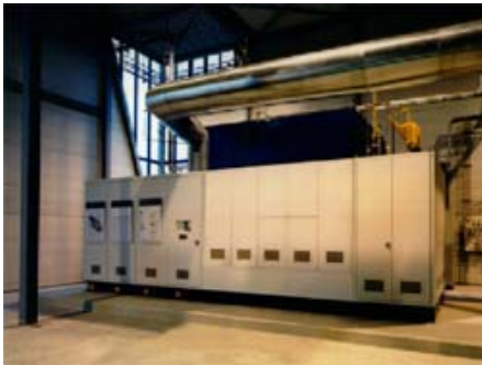
Sistema SOFC Westinghouse 100 kW
